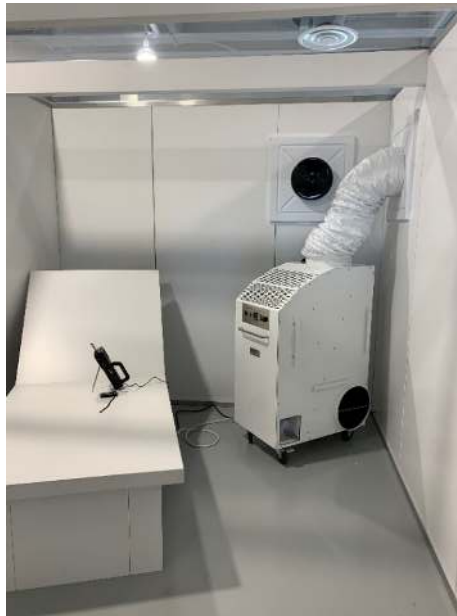
Figure 5: Room After Installation for Negative Pressure
