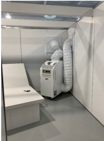
Figure 7: Room After Installation for Positive Pressure
